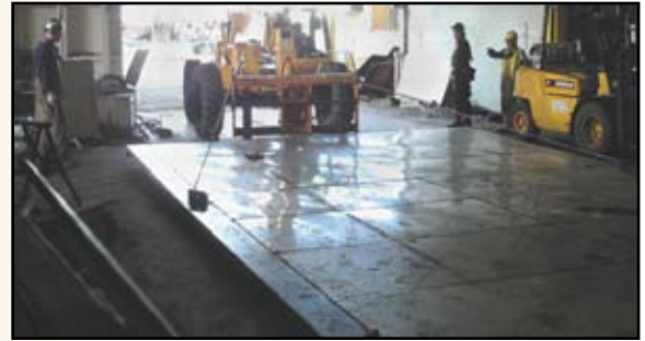
Above, a Westmill stainless steel floor module is pushed into a Dryer from the end.
