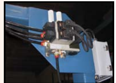
Pneumatic valves wired to junction box
