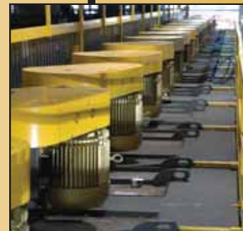
Hot air circulation fans
