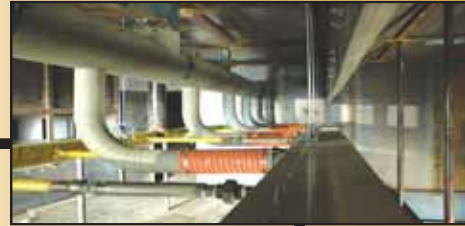
Gas piping/combustion air delivery piping
