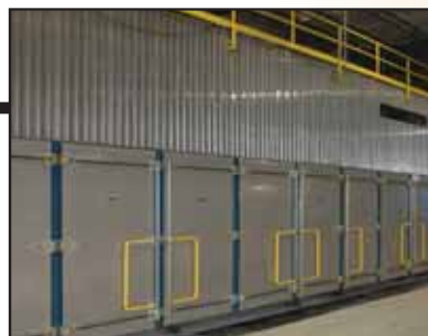
Dryer doors and handrail
