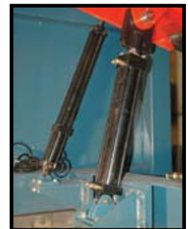
Hydraulic cylinders on new tipple
