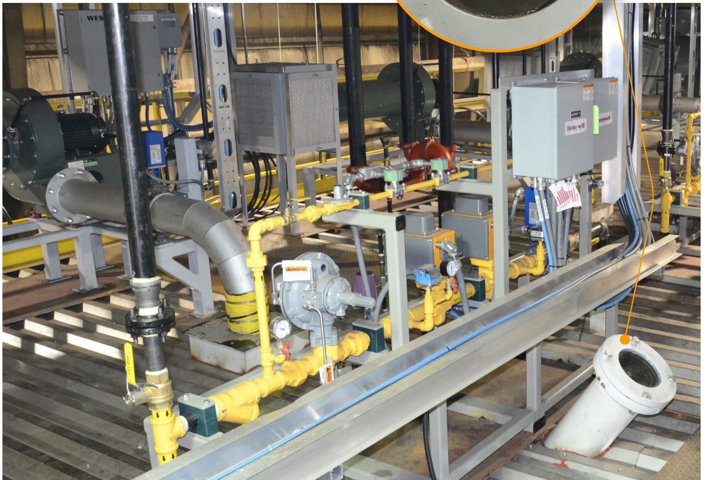
Westmill Dryer - Low NOx Gas Train
