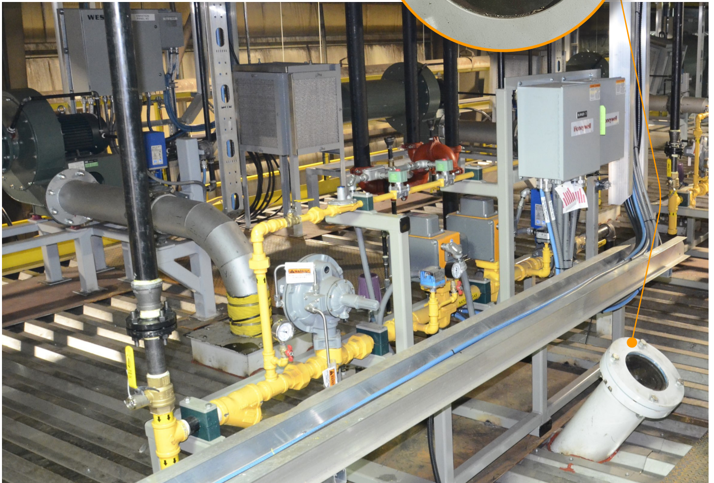
Westmill Dryer - Low NOx Gas Train
