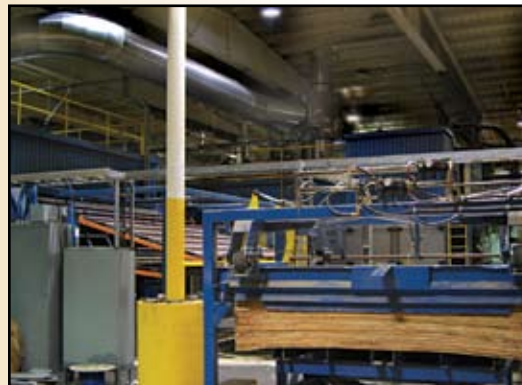
Heating duct from 6-Deck Longitudinal to a Screen Redryer.
