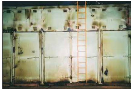
Doors and Side Panels - Before
