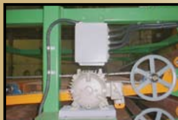
Individual Deck Drives with VFDs
