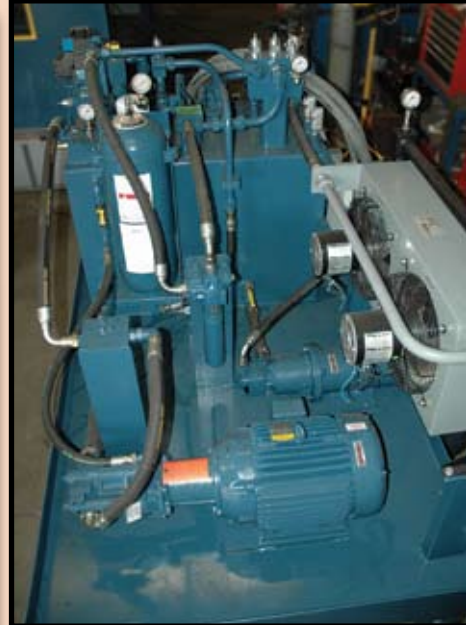
Westmill's Dryer Infeed Scissor Lift (far left) and Hydraulic Power Unit
