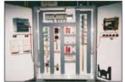
Dryer Control Panel - Inside
