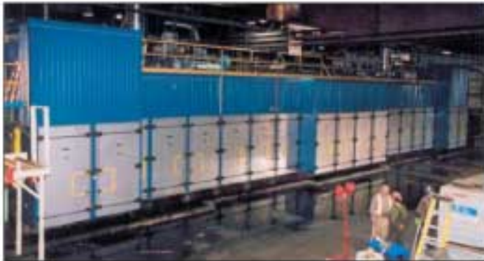
A Westmill Two-Zone Dryer remodel at Coastland Wood Industries, Delta, BC including Stainless Steel Insulated floor, PLC Dryer Controls, Gas Burners, Fans, Motors and VFD's, Humidity monitoring & Spray system - completed in 13 days!
