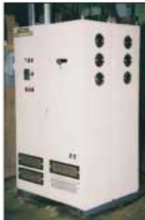
VFD Control Cabinet
